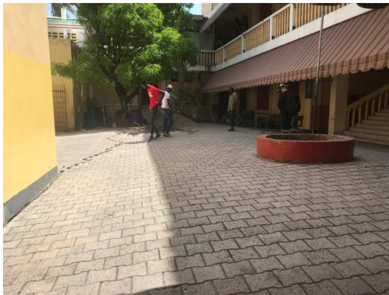
Figure 37 - Building 21 courtyard heave
