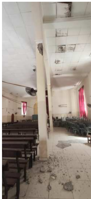
Figure 39 - Extensive structural cracking observed from inside the “auditorium” building
