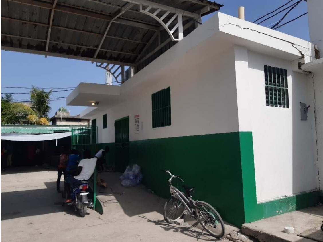
Figure 15 - Building 6, image shows cracking to the external edge of the roof slab
