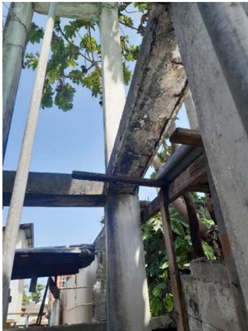
Figure 10 - Spalling of the concrete on the beam
