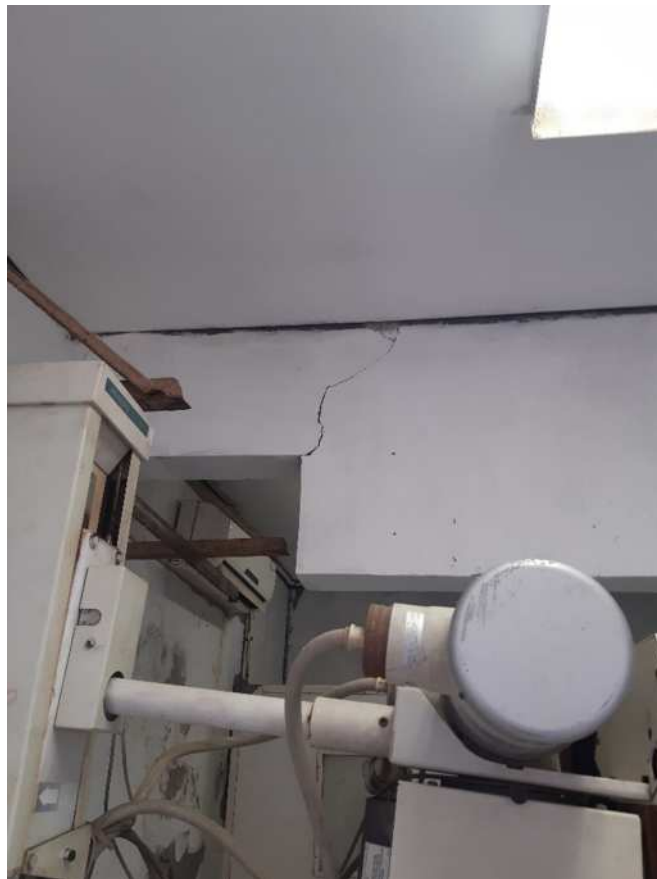
Figure 17 - Cracking of the supporting beam
