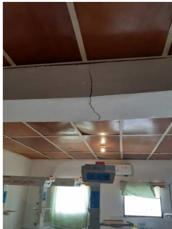
Figure 23 - Crack in a supporting beam
