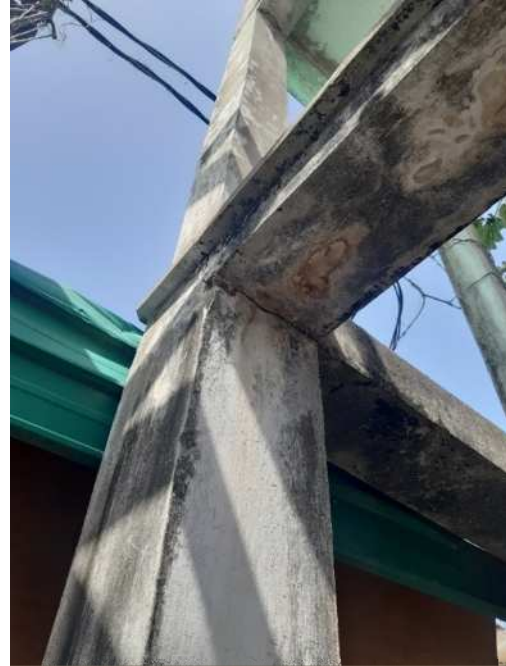
Figure 9 - Cracking between the beam and column joints
