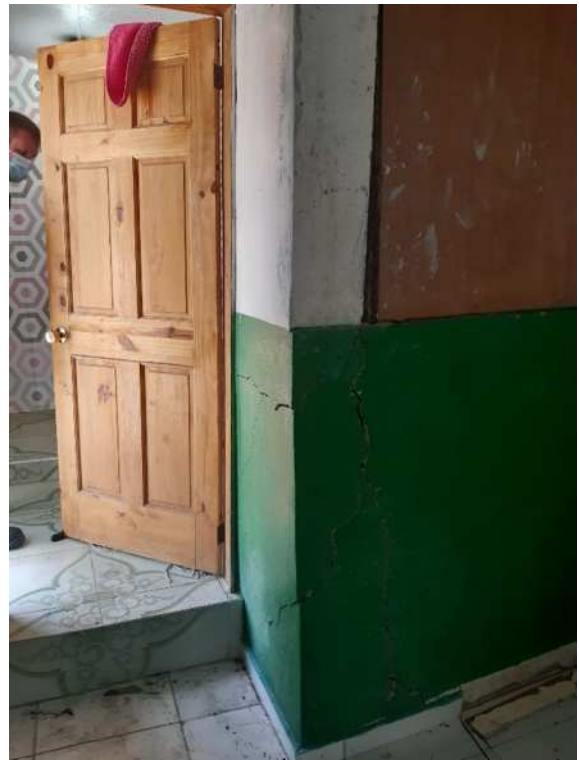
Figure 13 - Cracked and leaning wall in Building 5
