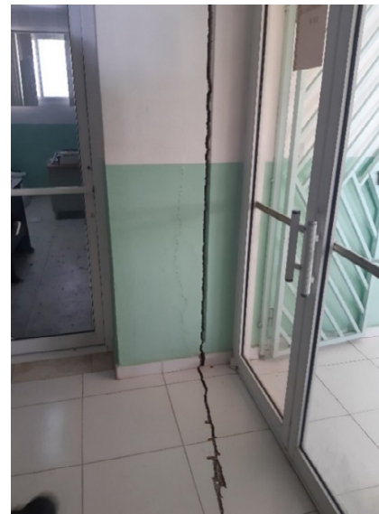
Figure 68 - Movement joint cracking
