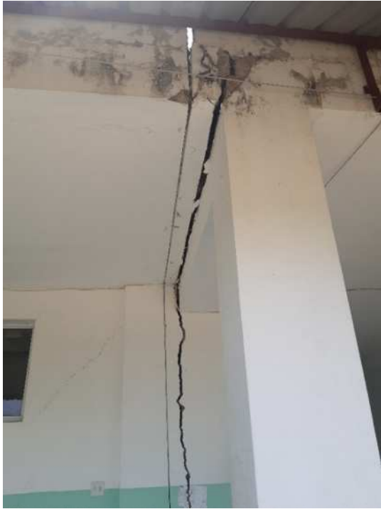
Figure 69 - Movement joint cracking resulting in loose fill
