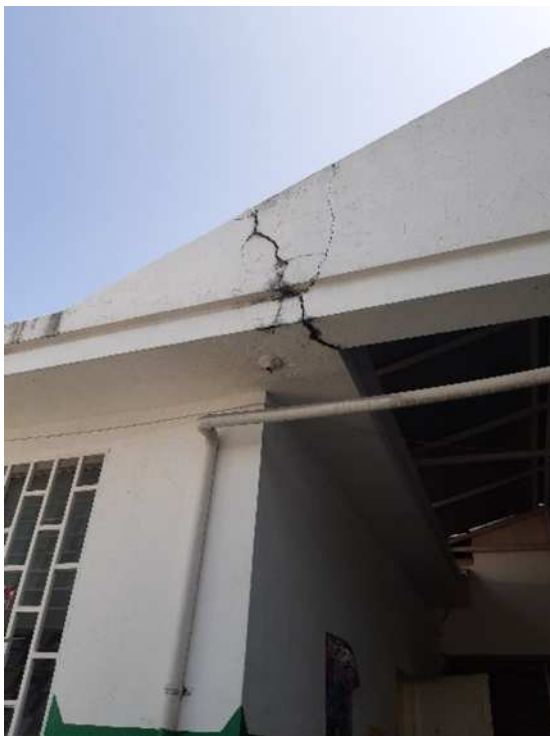
Figure 22 - Crack in the entrance arch
