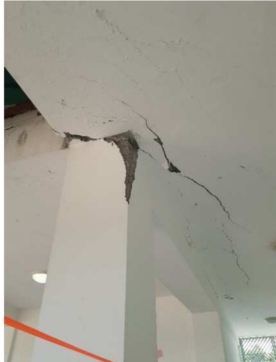
Figure 70 - Cracking around the column head and slab
