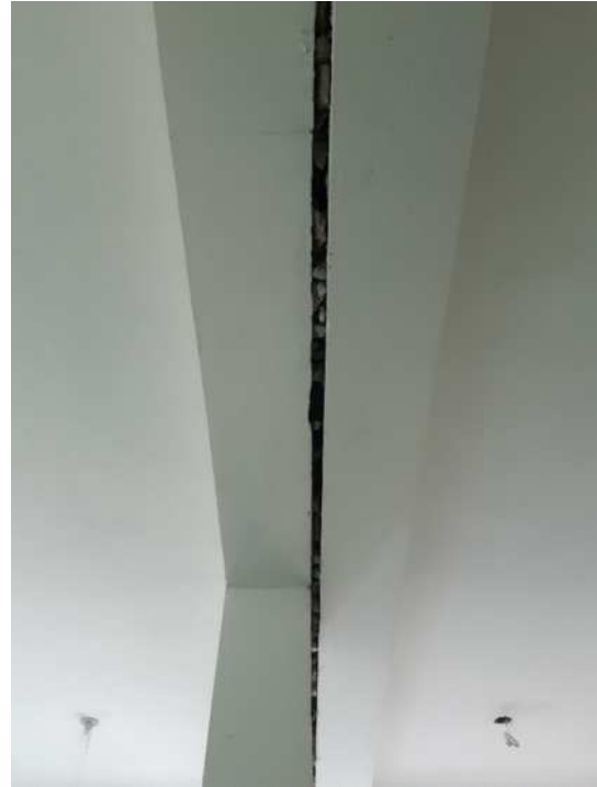
Figure 30 - Cracking along the movement joint in building 15
