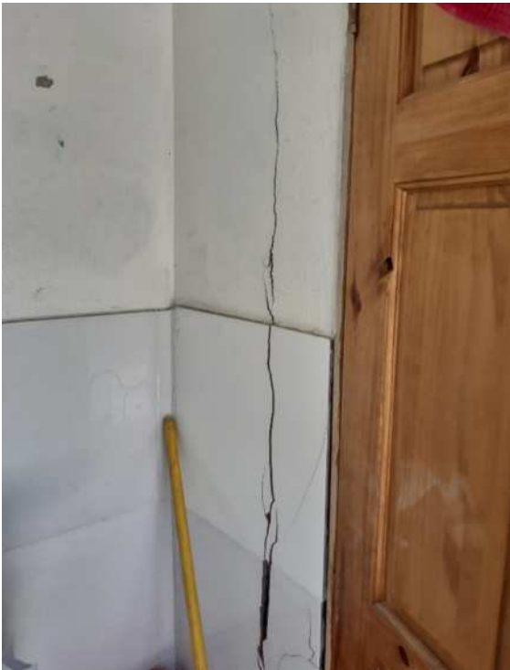
Figure 12 - Cracked and leaning wall in Building 5
