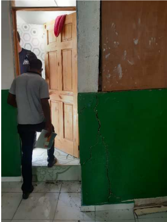
Figure 14 - Cracking observed on the opposite side of the wall shown above
