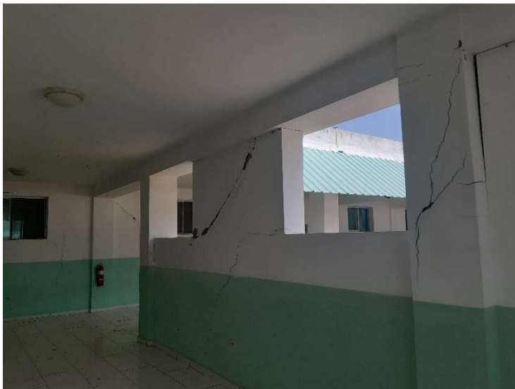
Figure 71 - Column cracking and short column shear crack
