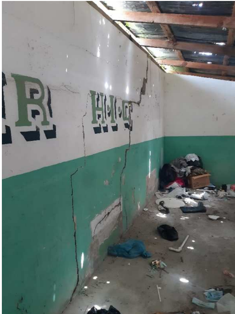
Figure 11 - Building 4, cracks in the rear wall
