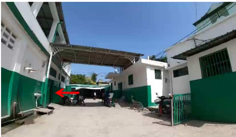
Figure 6 - Access into the room with a damaged column is indicated by the red arrow.
