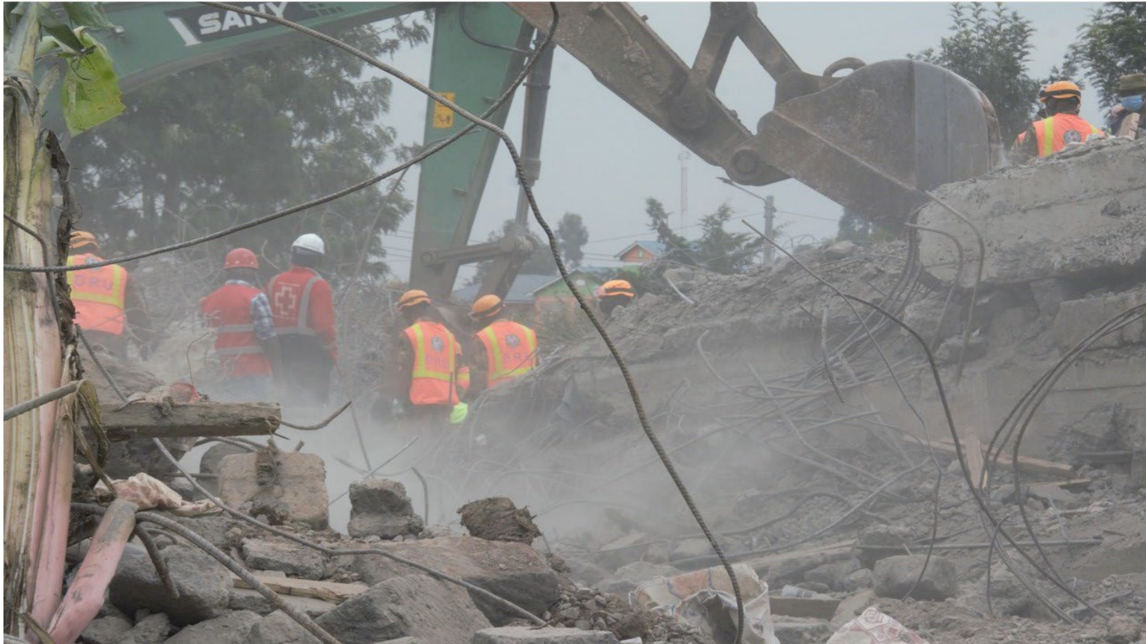
GACHIE Building Collapse 23rd Sept 2021
