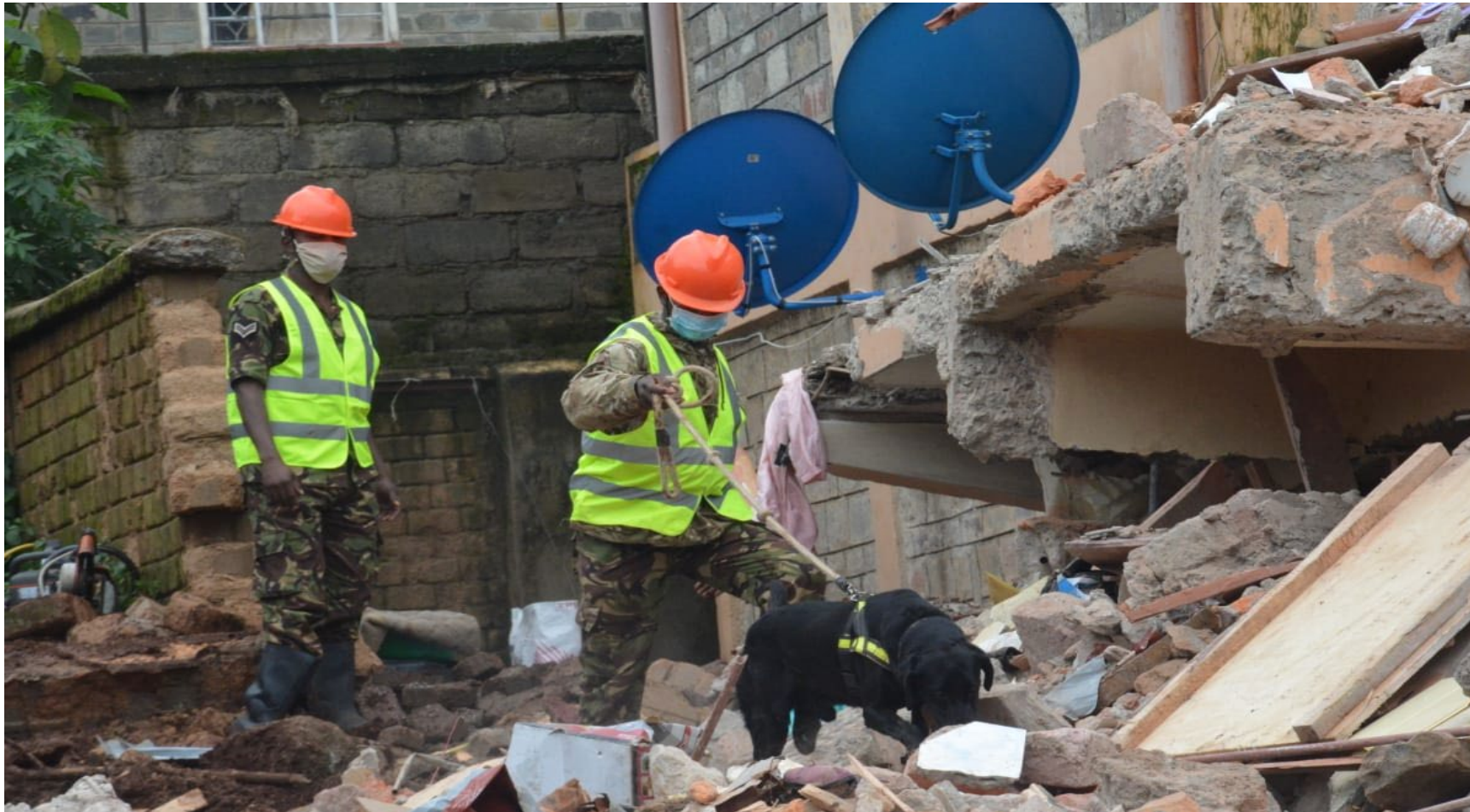
KERICHO Building collapse 2020
