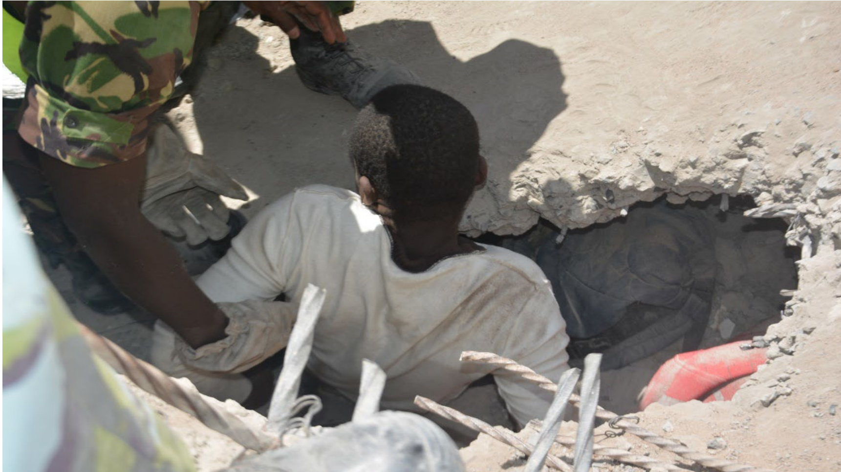
Tassia collapsed building 8 TH Dec 2019
